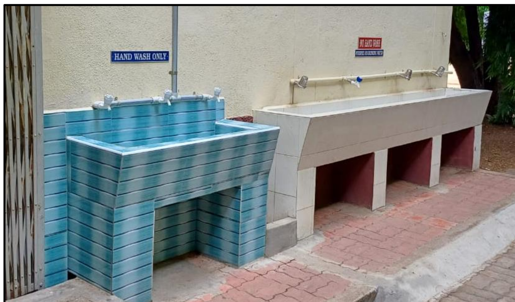
Proper Maintenance of Taps without any leakages in Sacred Heart College (Autonomous), Tirupattur, TN
