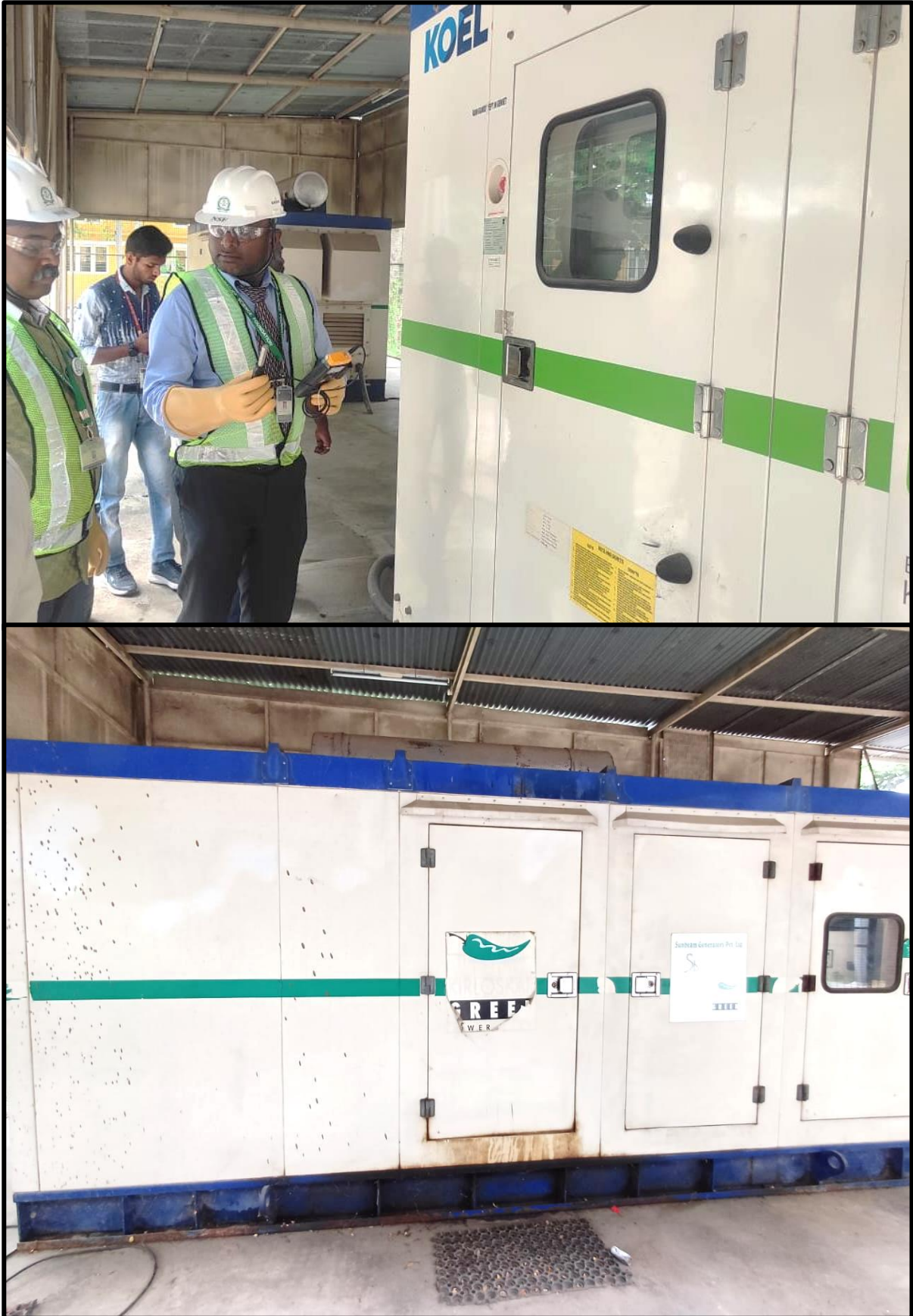
Generators Facility available in the Campus of Sacred Heart College (Autonomous), Tirupattur, TN
