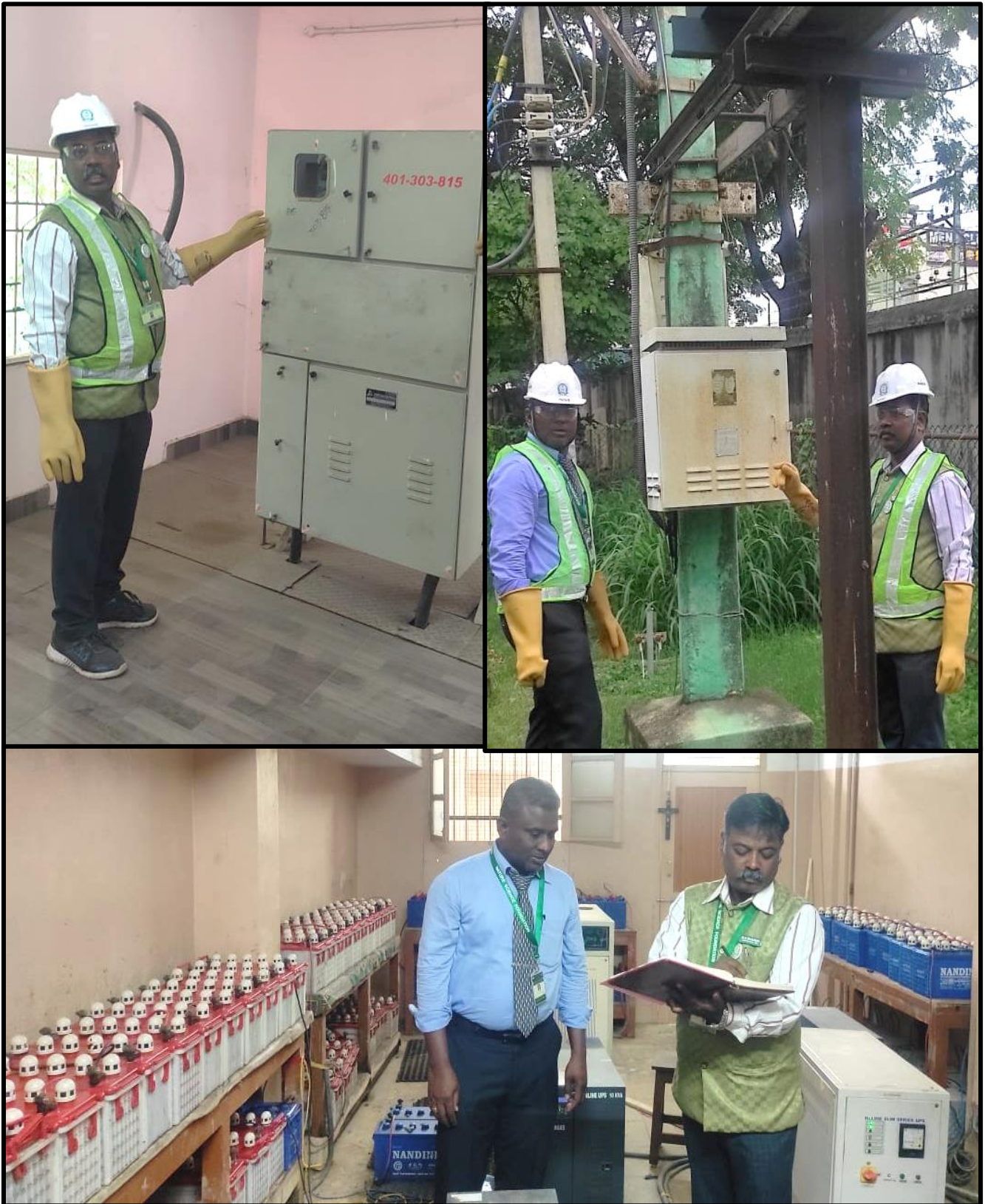
Transformer, UPS and Power Rooms are well maintained in the Sacred Heart College (Autonomous), Tirupattur, TN
