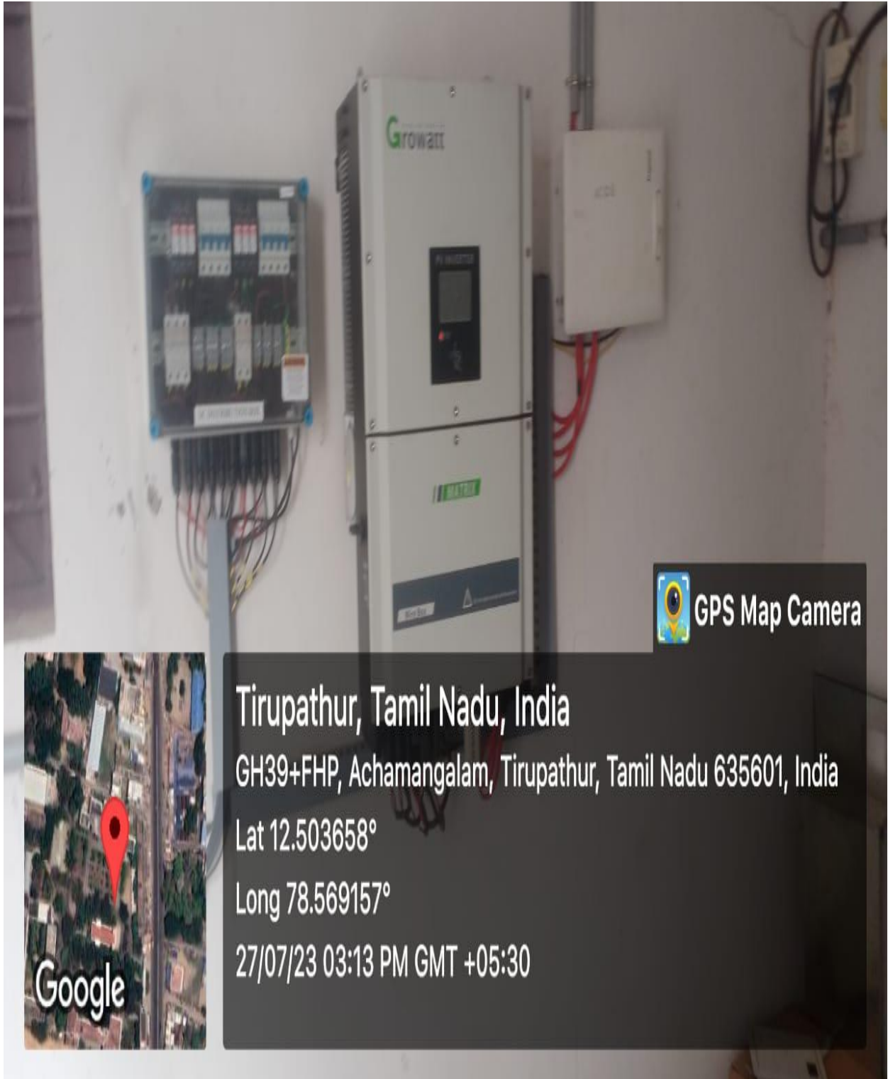
Connection to the Grid
