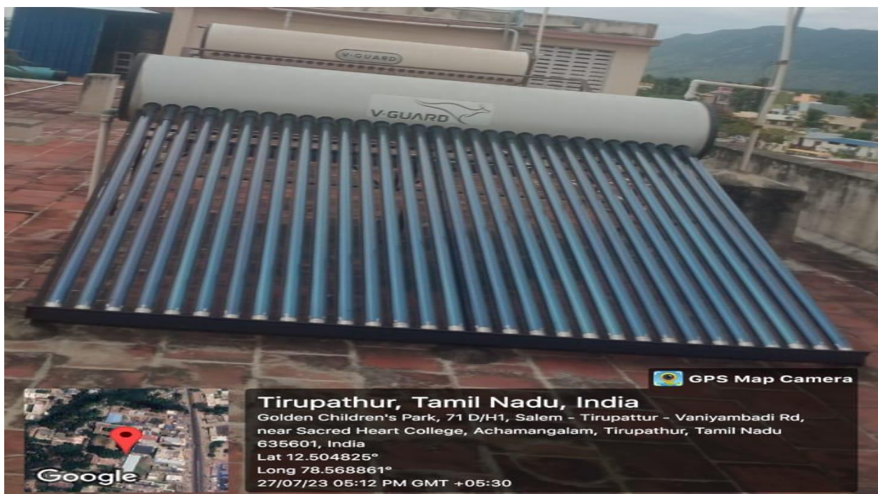
Solar Water Heater in the Terrace of Amalagam Hostel
